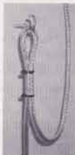
Fig. 5. Cable installation example
